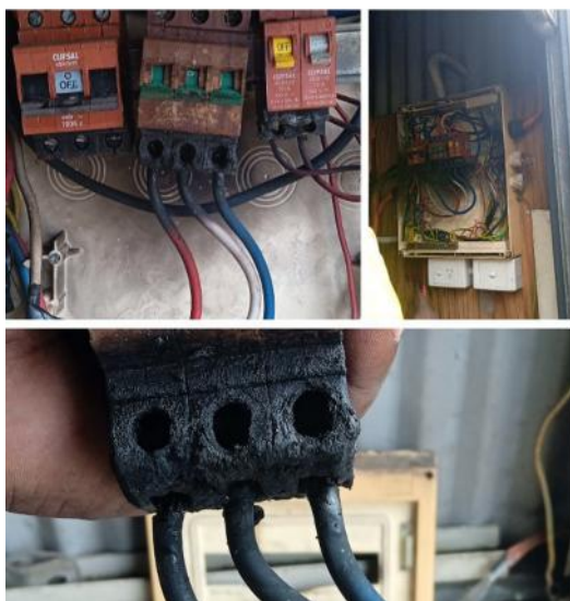
Figure 34: NAIC power damage
